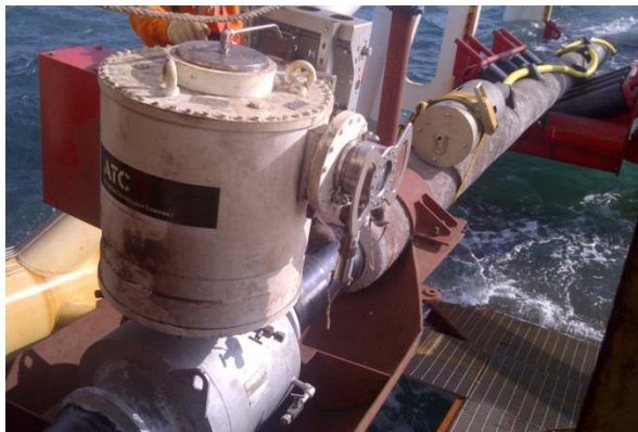
Rigid pipelay of about 150 KM with Midline tie-in of pipeline and Optic Fibre Cable,
